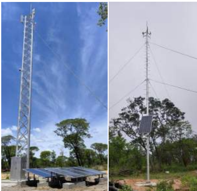
5G base station powered by photovoltaic energy storage
