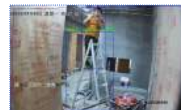
Elevated work without safety belt
